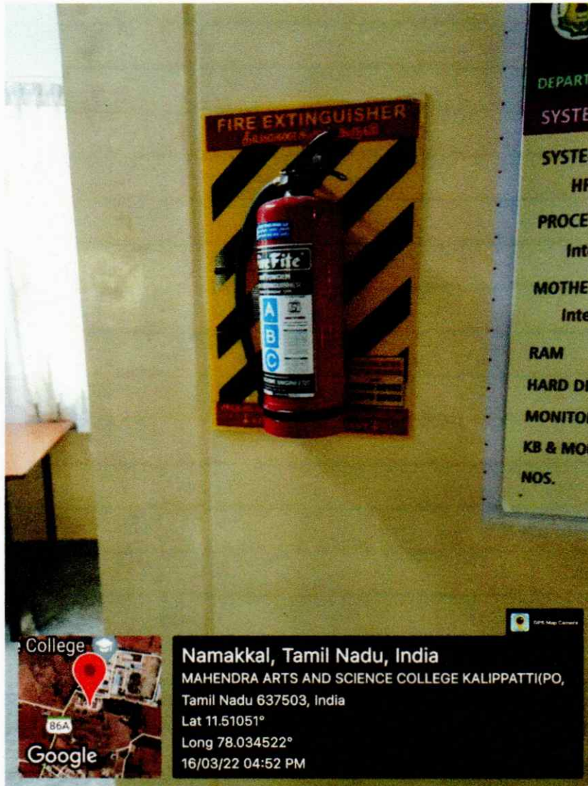
FIRE EXTINGUISHER IN ROUND BLOCK I FLOOR
